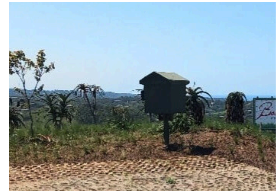
Invertors x 4 Installed
